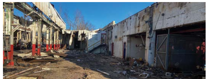
The remains of Allsource Logistics after a tornado swept through Dawson Springs, Kentucky.
